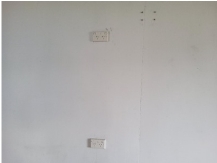
Photo uploaded: Building 3 Power outlets 18 Dec 2023 1:09pm
