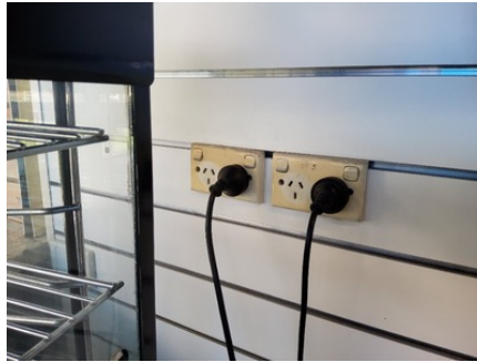
Photo uploaded: Building 1 Power outlets 18 Dec 2023 12:26pm
