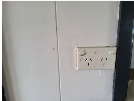
Photo uploaded: Building 3 Power outlets 18 Dec 2023 1:08pm
