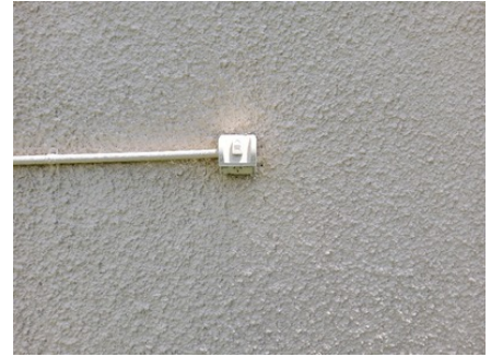
Photo uploaded: Building 3 Power outlets 18 Dec 2023 1:09pm
