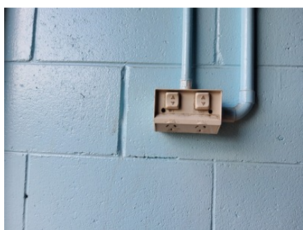
Photo uploaded: Building 2 Power outlets 18 Dec 2023 12:45pm
