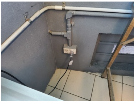
Photo uploaded: Building 1 Power outlets 18 Dec 2023 12:26pm
