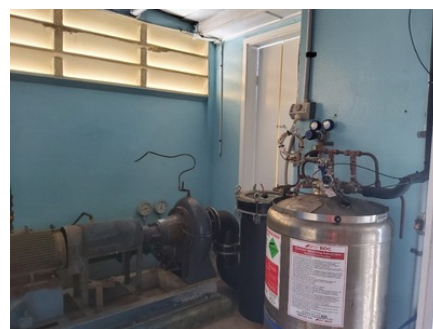
Photo uploaded: Building 2 Utilities/plant room 18 Dec 2023 12:42pm
