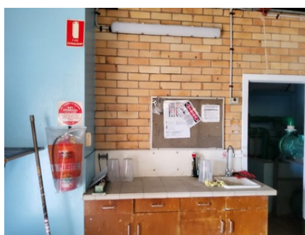
Photo uploaded: Building 2 Power outlets 18 Dec 2023 12:45pm
