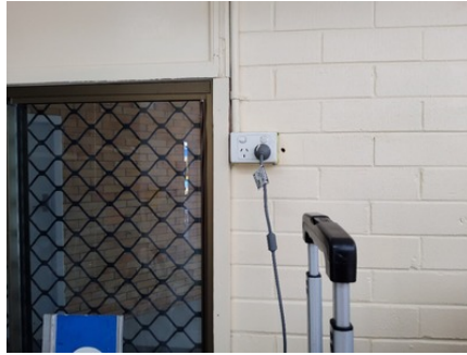
Photo uploaded: Building 1 Power outlets 18 Dec 2023 12:27pm
