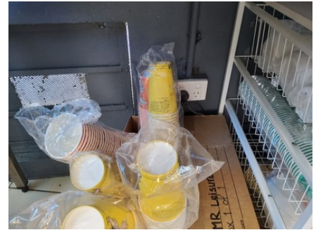
Photo uploaded: Building 1 Power outlets 18 Dec 2023 12:26pm
