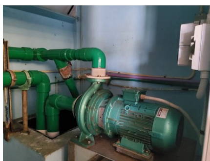
Photo uploaded: Building 2 Utilities/plant room
