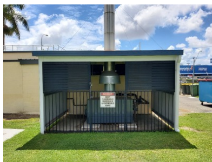
Photo uploaded: Building 2 Utilities/plant room 18 Dec 2023 12:42pm
