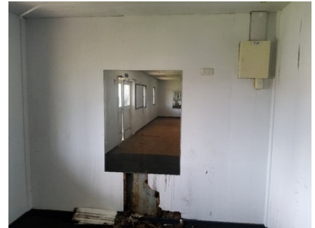
Photo uploaded: Building 3 Power outlets 18 Dec 2023 1:08pm
