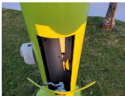
Photo uploaded: Supporting Amenities 1 Outdoor power supply 20 Oct 2023 6:54pm
