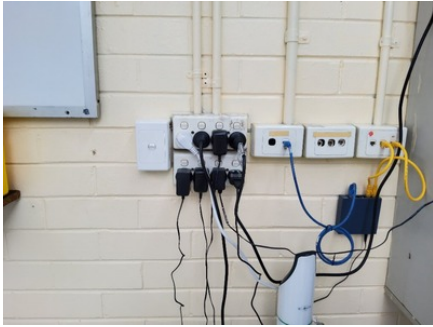
Photo uploaded: Building 1 Power outlets 18 Dec 2023 12:28pm
