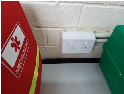
Photo uploaded: Building 1 Power outlets 18 Dec 2023 12:27pm
