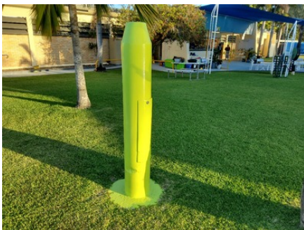
Photo uploaded: Supporting Amenities 1 Outdoor power supply 20 Oct 2023 6:17pm
