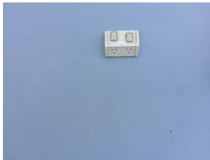
Photo uploaded: Building 1 Power outlets 11 Oct 2023 3:32pm
