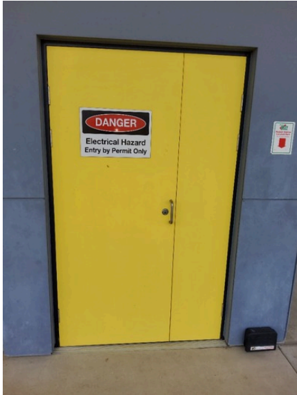
Photo uploaded: Building 2 Utilities/plant room 12 Oct 2023 12:33pm
