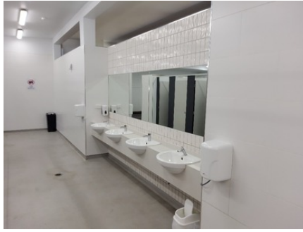
Photo uploaded: Supporting Amenities 1 Spectator toilets 11 Oct 2023 1:45pm
