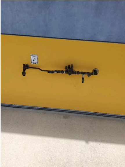
Photo uploaded: Building 2 Rainwater storage 12 Oct 2023 12:44pm Nonpotable water.
